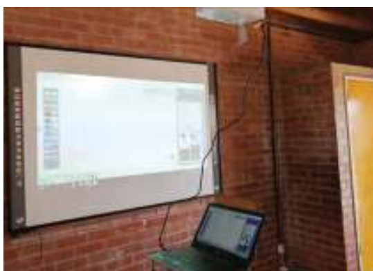
A digital board and projector installed by FBC at Mawaba Primary School in Bulawayo.
